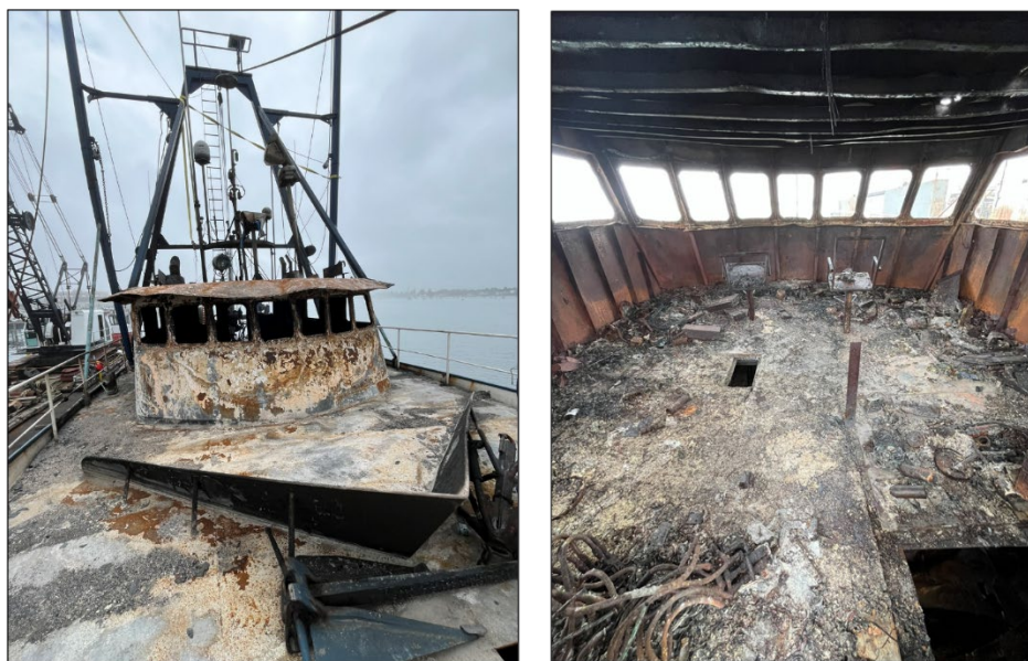
Figure 5. Left to right: Foredeck of the fishing vessel Three Girls after the fire, and fire damage to the interior of wheelhouse after the fire.
