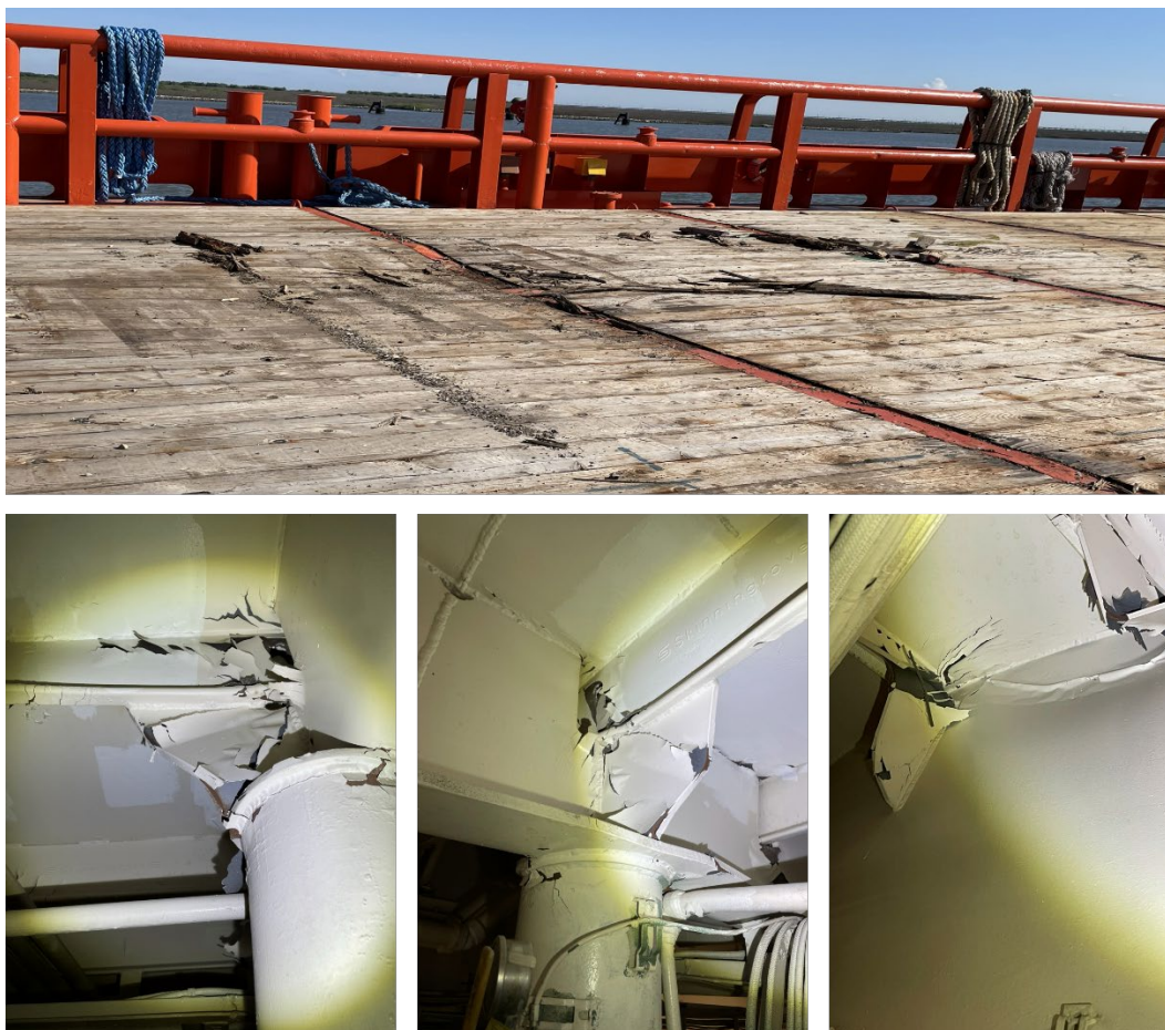
Figure 5. Damage to C-Enforcer main deck (top) and framing of upper engine room and liquid mud tank (below).
